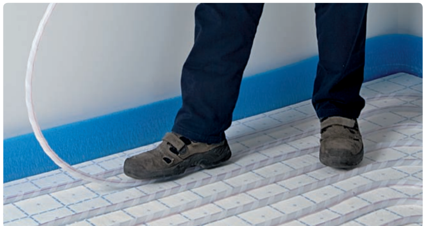
Reposition the pipe and secure in place by simply treading on it again. You can also lift and refix using your hands
