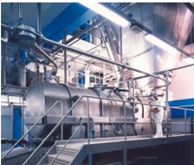
Certain industrial / commercial applications require high levels of hygiene, such as this Dairy Facility shown above. The Inox Ultra pro with it's all Stainless Steel construction and fully potable / alimentary membrane is the ideal selection in such an environment.
